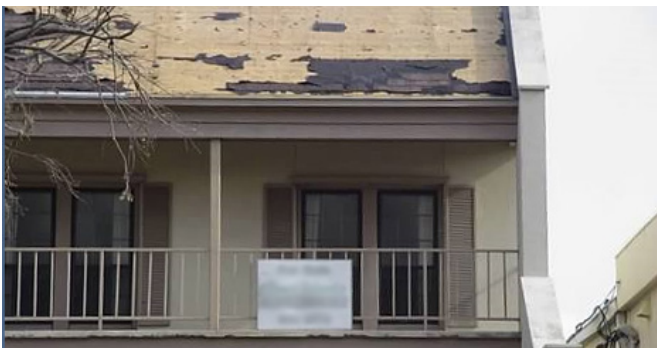
Figure 3 - Visual Image of Damaged Roof
