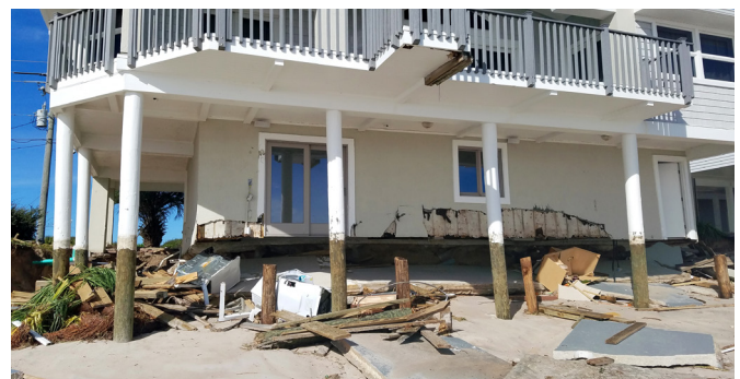
Figure 1 - Visual Image of Exterior Structural Damage
