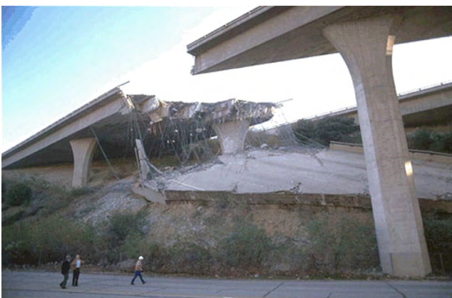
Photo 3 - A destroyed segment of the I-5 Freeway in Northridge, California; 1994 (Credit: FEMA/Wikimedia Commons )
