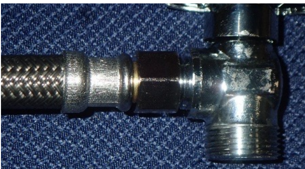
Flexible connector installed on shut off valve
