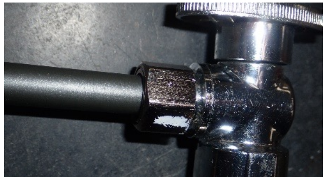
Preassembled compression connector installed
